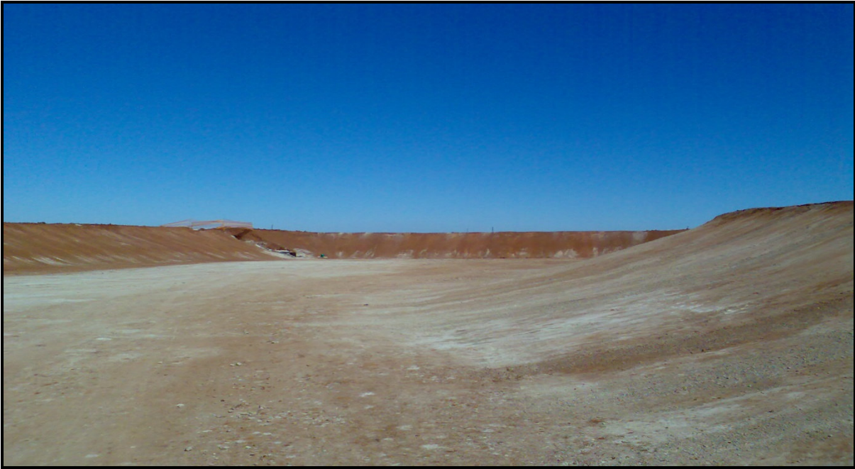
Figure 15: Some more earthworks being carried out on disturbed mining land (Rossouw 2008: Isibonello Colliery)
