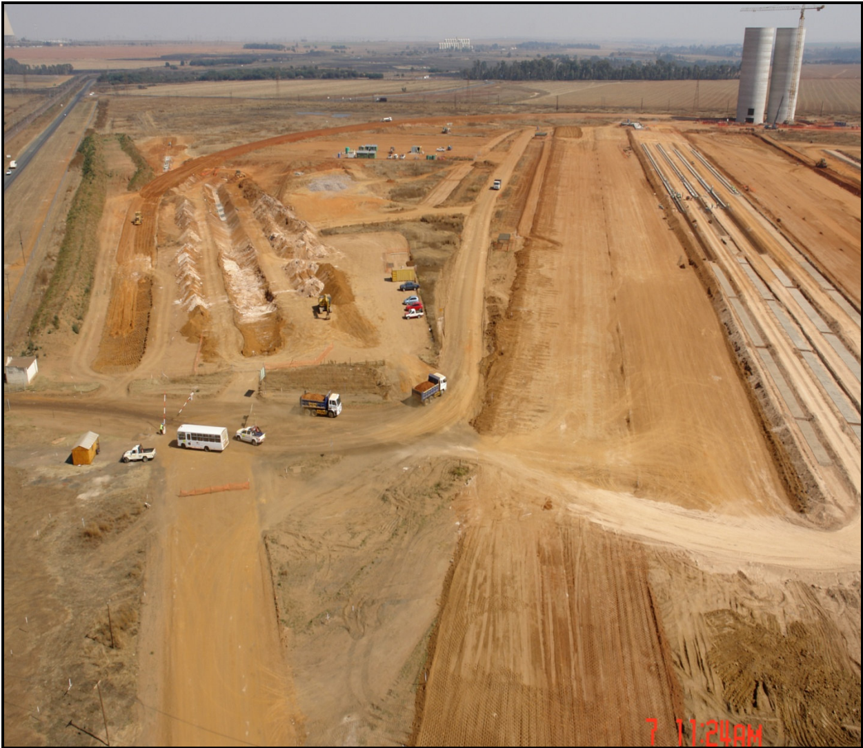
Figure 4: The terraces and earthworks being constructed for new buildings that will be built on the coal mine
