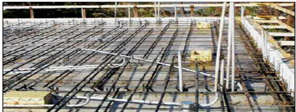
Figure 15: Photo of slab formwork, reinforcement bars and electrical conduits ready for casting of concrete. (Source: concrete-forms.blogspot.com)
