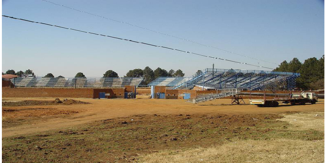
Figure 11, Taryn Eliot, Training for Township Initiative, 2007, illustrates the stadium upgrades to the HM Pitje Stadium in Mamelodi West
