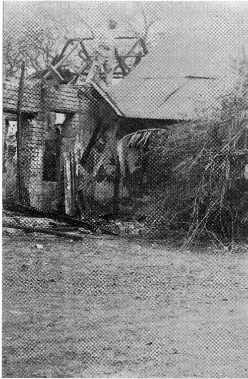
In 1955 the Bras Perreira house was demolished. Photos show demolition work in progress.
