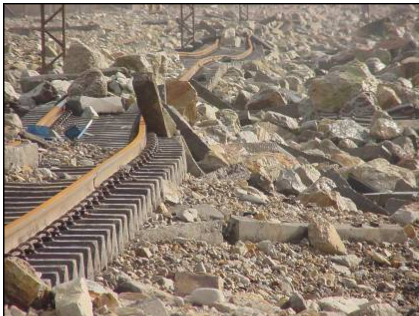
Figure 9: Damage to the Railway Line
