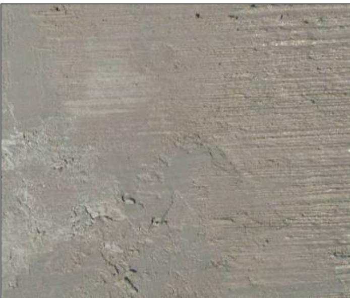
Photo 11: Damage to texture due to plastic cover sheeting
