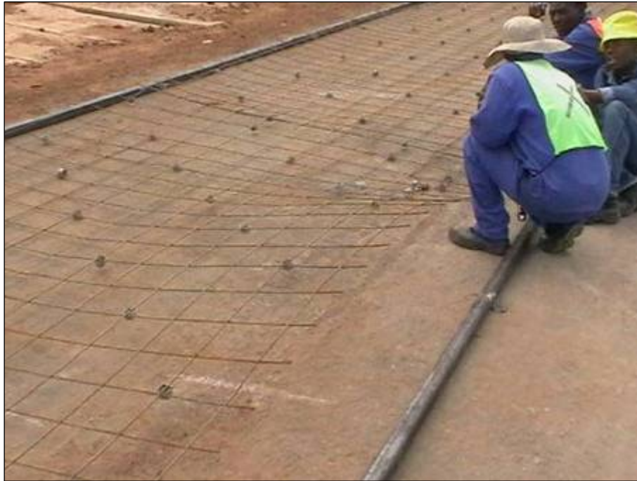
Photo 5: Mesh reinforcement damaged during transport
