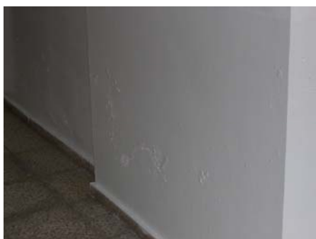
Figure 9: Blistering on a painted surface.
