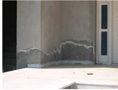
Figure 6: Efflorescence due to rising damp
