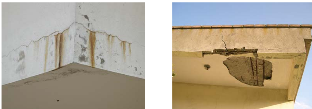
Figure 3: Corrosion of steel.
