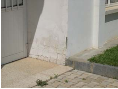
Figure 5: Render damage due to rising damp.
