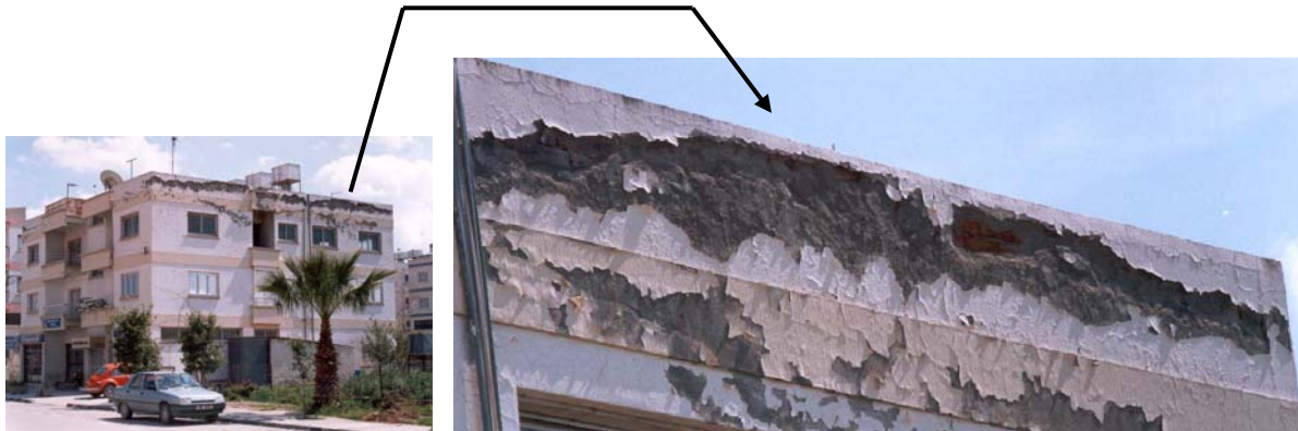
Figure 7: Deteriorations on the concrete surfaces.
