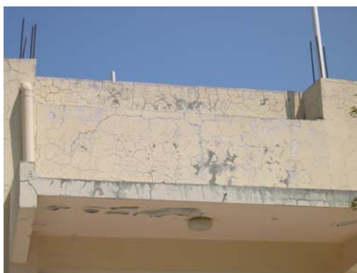
Figure 4: Craze type of cracks.
