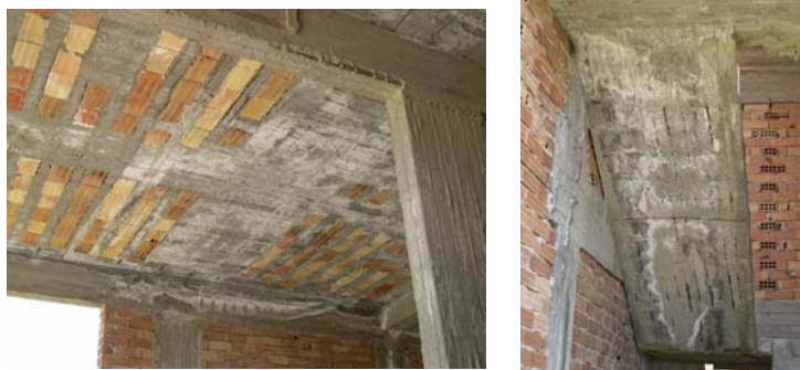
Figure 8: Efflorescence on the concrete surfaces.
