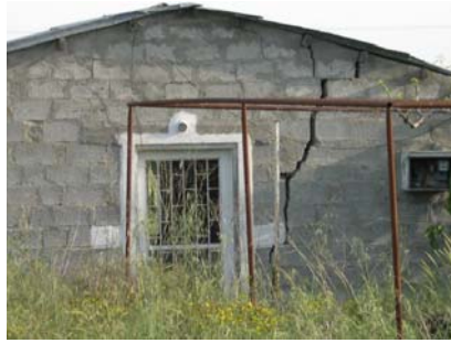
Figure 1 : Crack on the building surface (left side) and on the plain concrete on the ground (right side).
