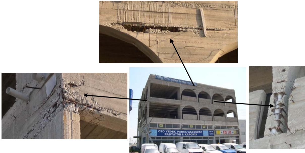
Figure 2: Honeycombing and compaction problems.
