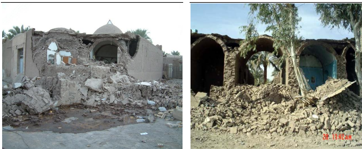
Figure 1: Extensive destruction of adobe buildings due to weakness of materials against lateral forces
