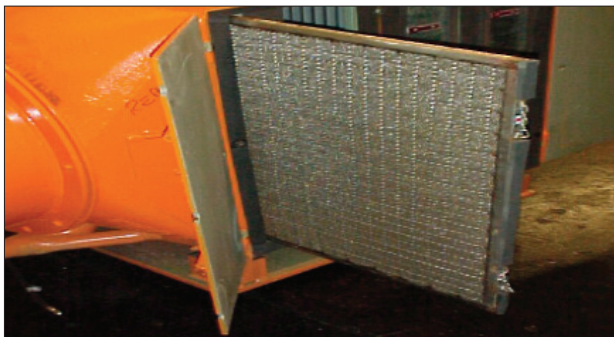
Figure 26—The filters of the scrubber
