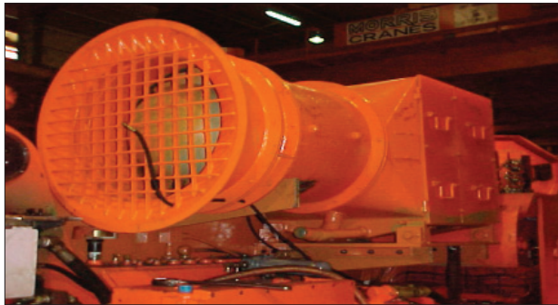
Figure 25—A scrubber unit
