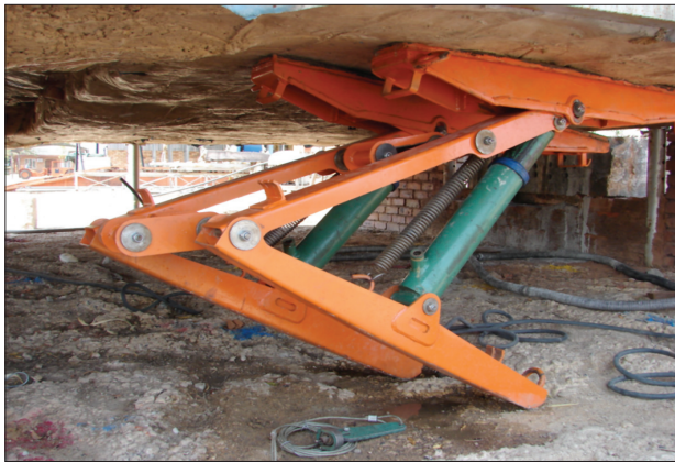
Figure 7—Photo of technology demonstrator roof support system in mock-up stope
