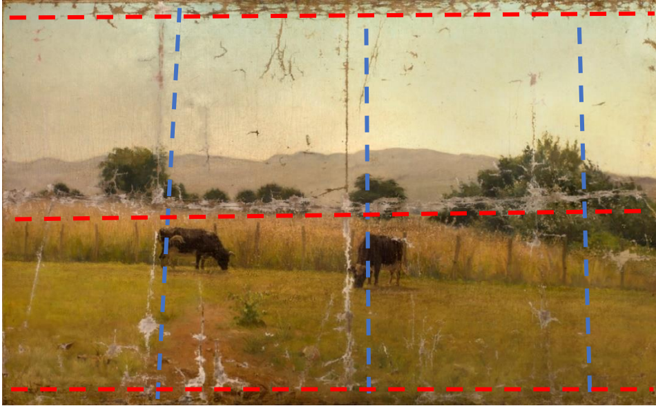
Figure 32: Major areas of paint loss along three horizontal folds (red stippled lines) and three vertical folds (blue stippled lines).
