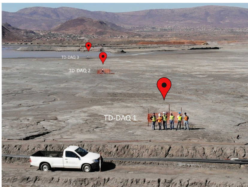
Fig. 13. UAV photograph of the three installed TD-DAQs.
