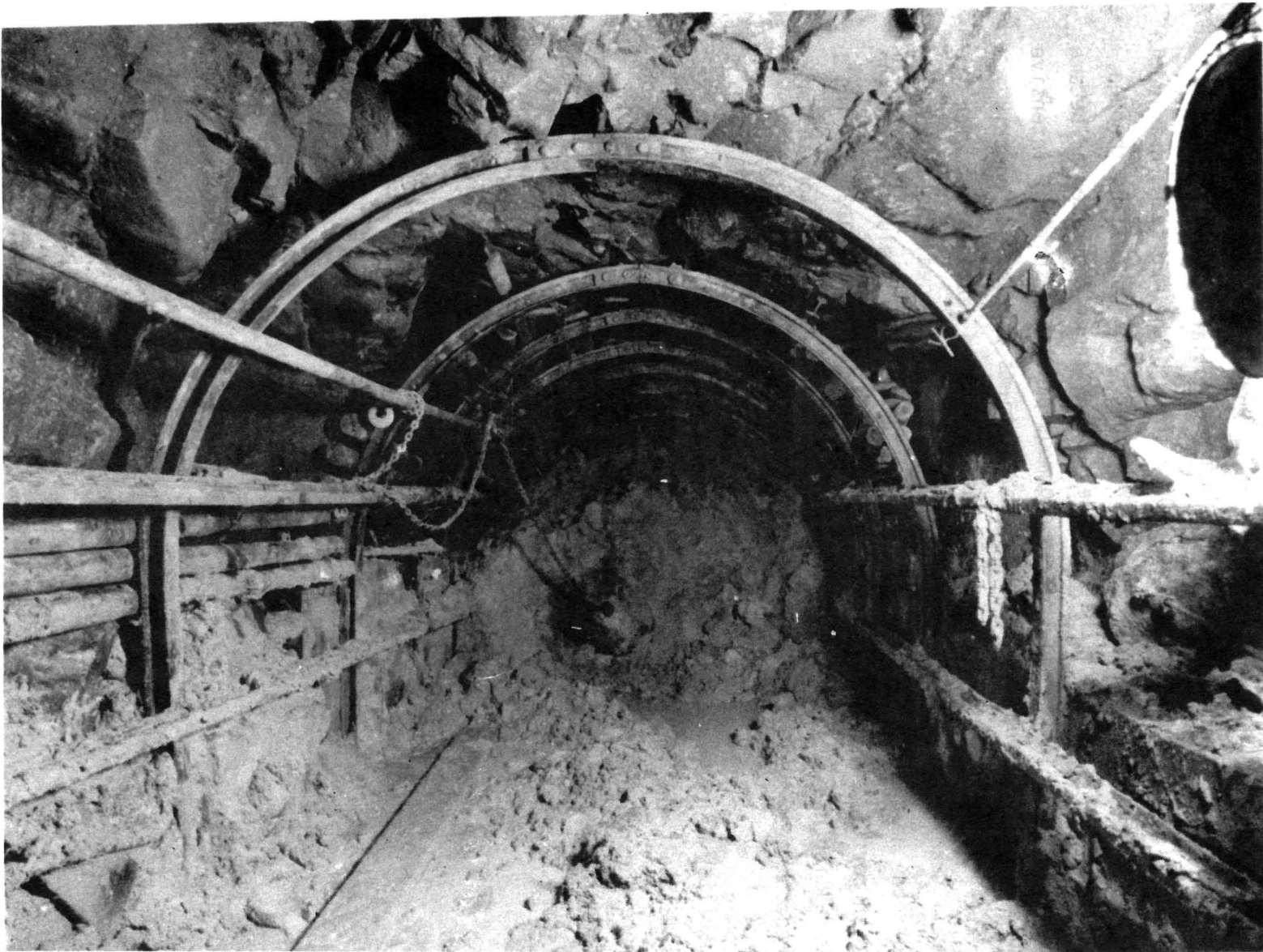
FIGURE 9/3 : Blockage in tunnel caused by mudrush from decomposed diabase dyke referred to in Figure 9/2.
