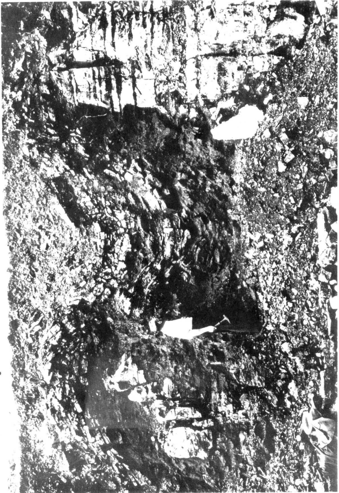
FIGURE 7/28 : Chert residuum sagging between pinnacles of dolomite in excavation for ore-bin at Vaal Reefs
