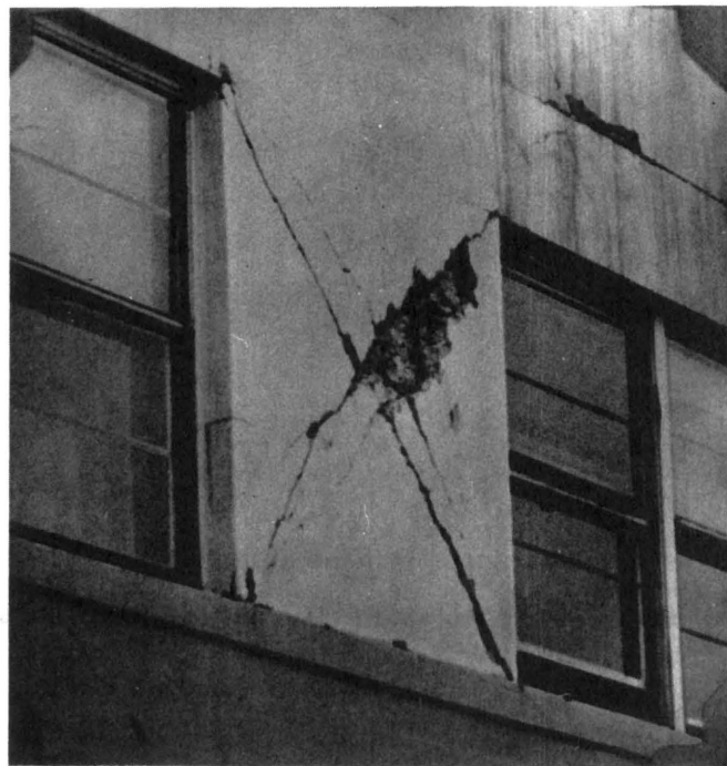
FIGURE 5/46 : Typical example of X-cracking induced by seismic waves in panel within beam and column frame ; building in Anchorage, after earthquake of 27.3.1964
