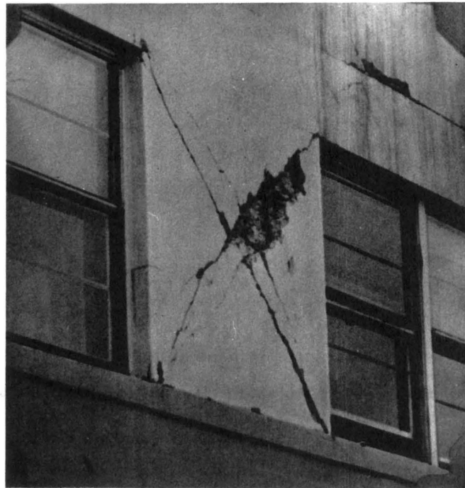
FIGURE 5/46 : Typical example of X-cracking induced by seismic waves in panel within beam and column frame : building in Anchorage, after earthquake of 27.3.1964
