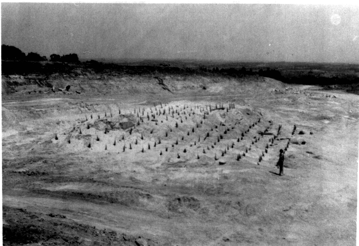
FIGURE 3/15 : Excavation for part of Johannesburg Western Bypass (Road N 1-20) showing core-stone-within residual granite
