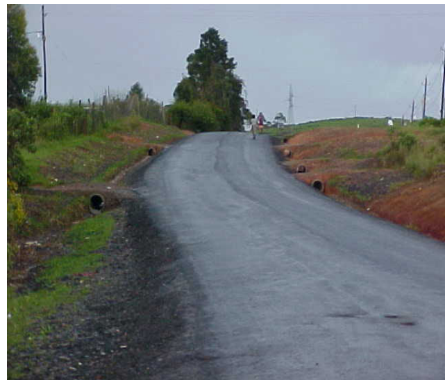
D 1132 Sweetwaters – Note Attention to Drainage, Accesses & Surfacing. Drainage Protection to follow.
