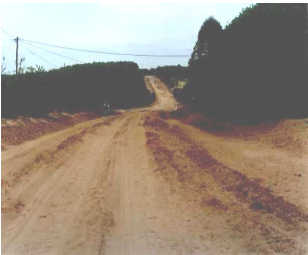
D 887 Before Upgrading – A poor sandy gravel road serving a large rural community and black sugar cane farmers.
