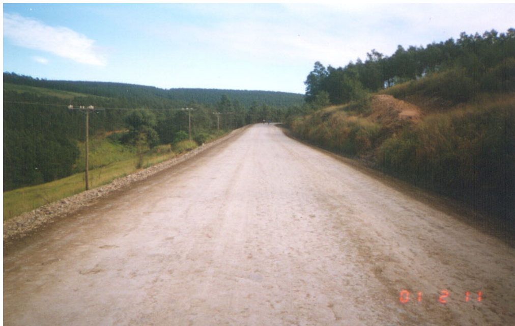
P 16/2 Kranskop – The C4 lime stabilised base preparation before the application of the cutback 150/200 penetration grade bitumen binder for the rural seal on the lime stabilised base layer.
