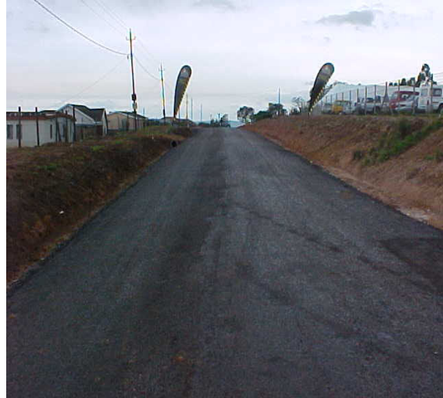
D1132 Sweetwaters – After upgrading with the application of a 150mm Rap base a hot prime and a 8mm thick slurry seal.
