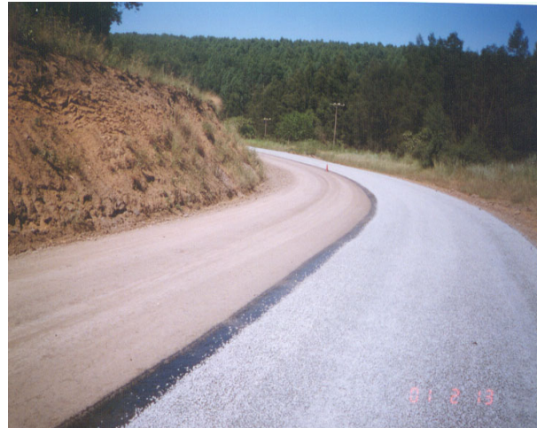
P 16/2 Kranskop - Application of half the cutback 150/200 penetration grade bitumen binder and the graded aggregate for the modified Otta seal. Note the exposed binder for the center joint overlap.
