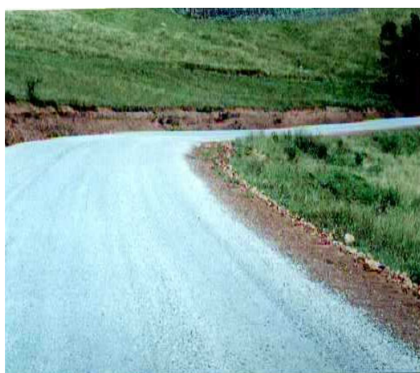
P50-2 NKANDLA; After Upgrading A low cost all weather road to serve the large rural community and give access to Nkandla.
