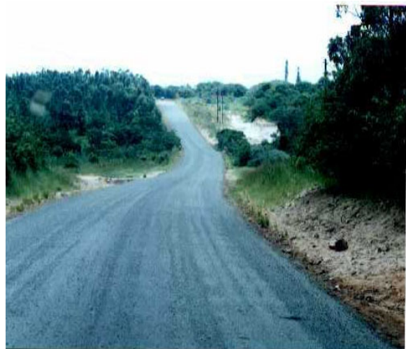
D 887 After Upgrading – A low cost all weather road to serve the large rural community and black sugar cane farmers.
