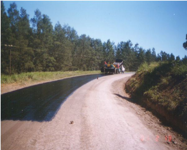
P 16/2 Kranskop - Application of the cutback 150/200 penetration grade bitumen binder for the modified Otta seal on the lime stabilised base layer.
