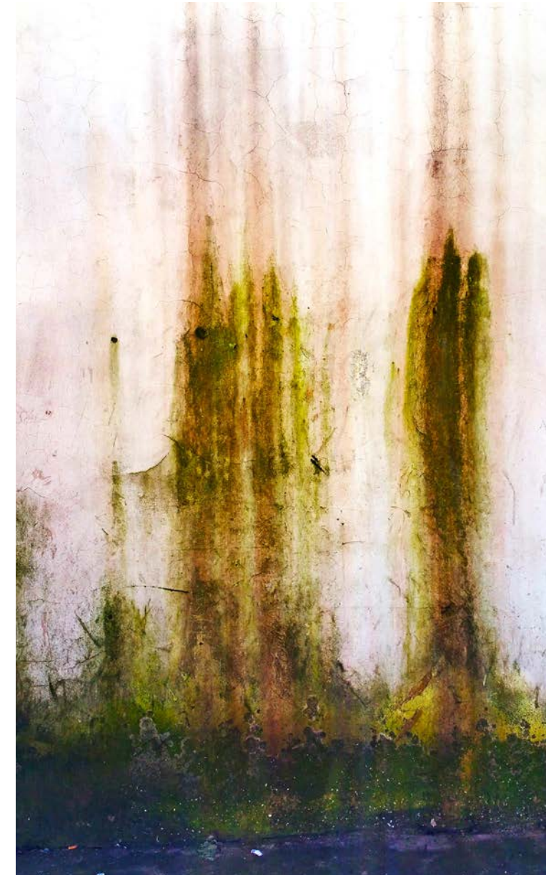
Fig.26. Weathering of a wall along Boom Street.
