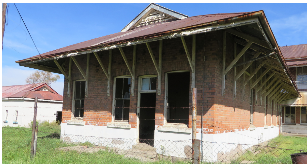
02.05: The NZASM Volksrust recreation hall (NZASM_SEL_003), which housed a kitchen for serving meals. The building, now abandoned, contains much valuable and original fabric and has high potential for re-use.
