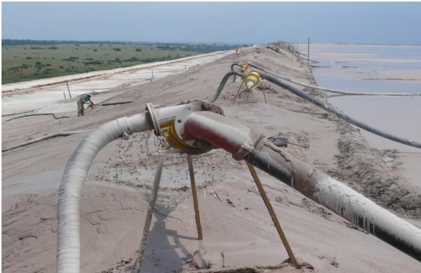
Figure 3.4: Chemwes Dam 5 hydrocyclones depositing underflow on dam wall
