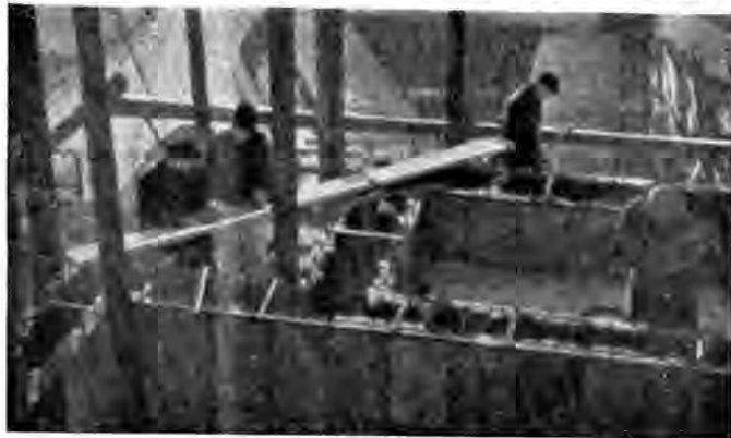
A building with Philipp Holzmann wall panels under construction. No shuttering is required, and considerable savings in labour, material and time are claimed.
