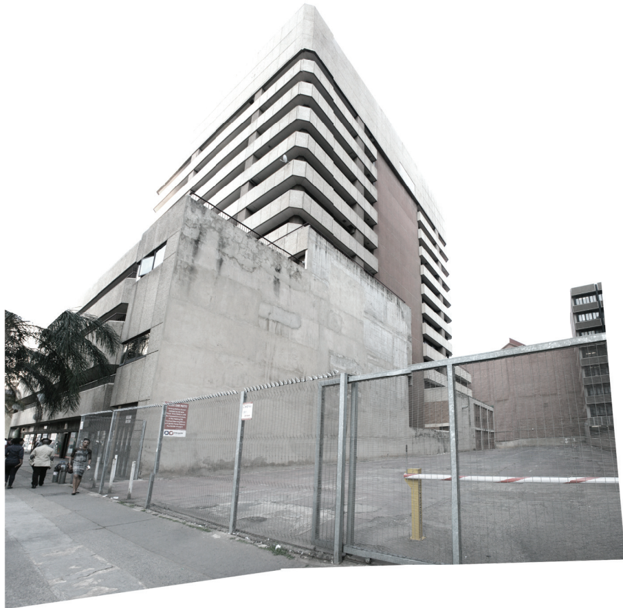
Figure 2.35 Eastern edge of the site. Unfinished concrete walls behave as membranes between the interior and exterior (Source: Author, 2015)
