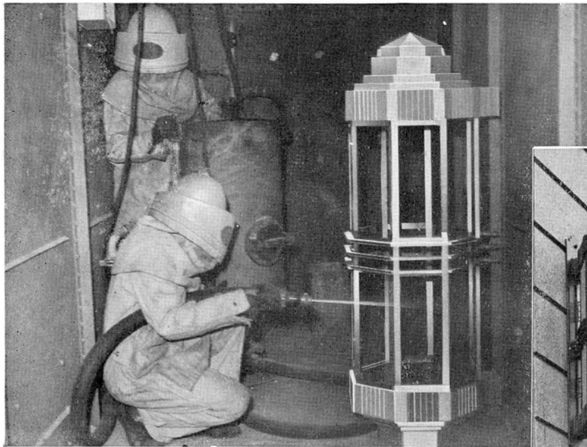
The lantern for the SOUTH AFRICAN MUTUAL BUILDINGS, Johannesburg, is shown during the process of sandblasting and also when completed and erected.
