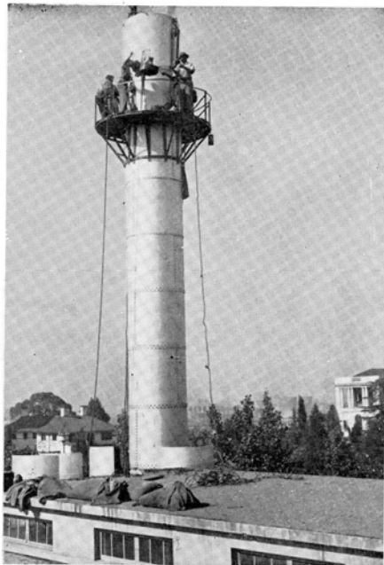
(Top) Construction of 125-foot steel self-supporting smoke stack supplied for General Hospital boiler house.
