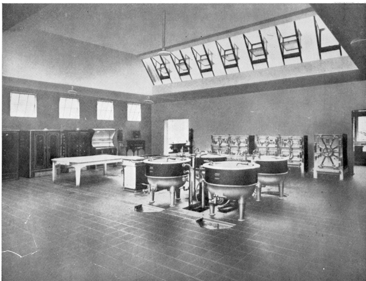
The photograph above shows typical Ashwell & Nesbit equipment recently installed in a modern Kitchen of a large hospital. The apparatus is finished in grey mottled enamel.
