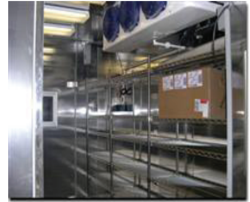
Figure 78: Cooler and freezer room
