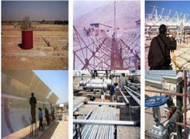
Figure 3 Installation of heat exchangers, valves, mirrors and absorber tube of Shiraz Solar Power Plant
