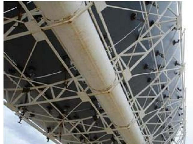
Figure 6 View of collector from back side
