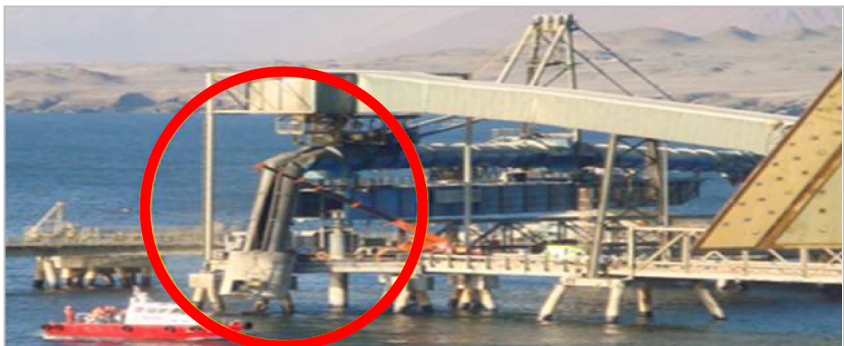
Figure 3.11: Ship loader, partially collapsed.
