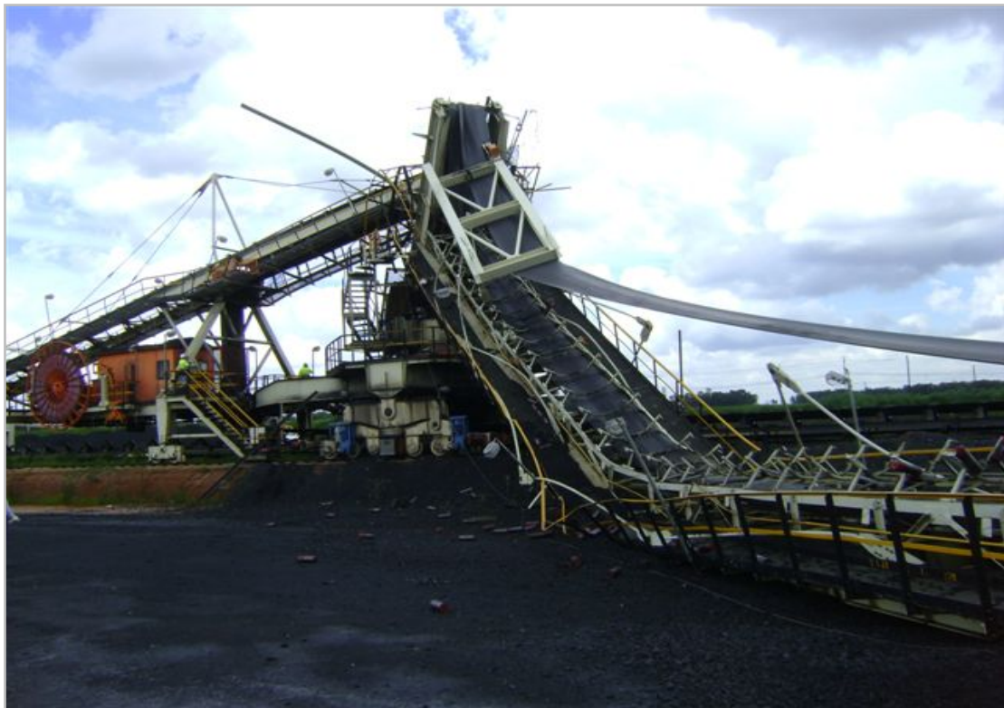
Figure 5.2: Collapsed stacker viewed from the north.
