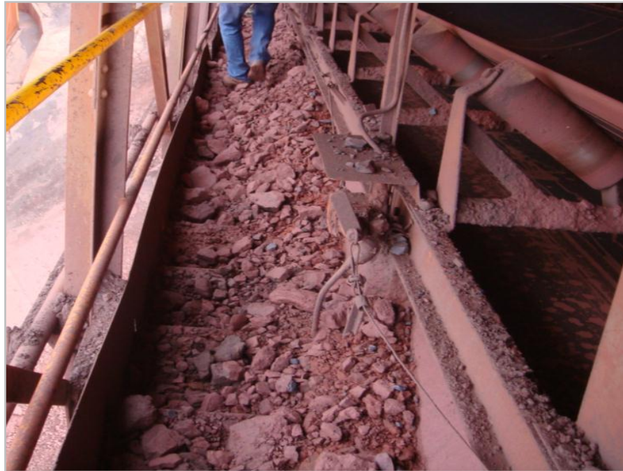
Figure 2.1: Conveyor walkway spillage.
