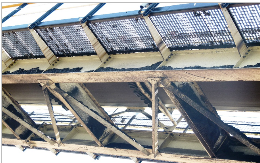
Figure 5.18: Scrape marks at the bottom of a stacker boom.
