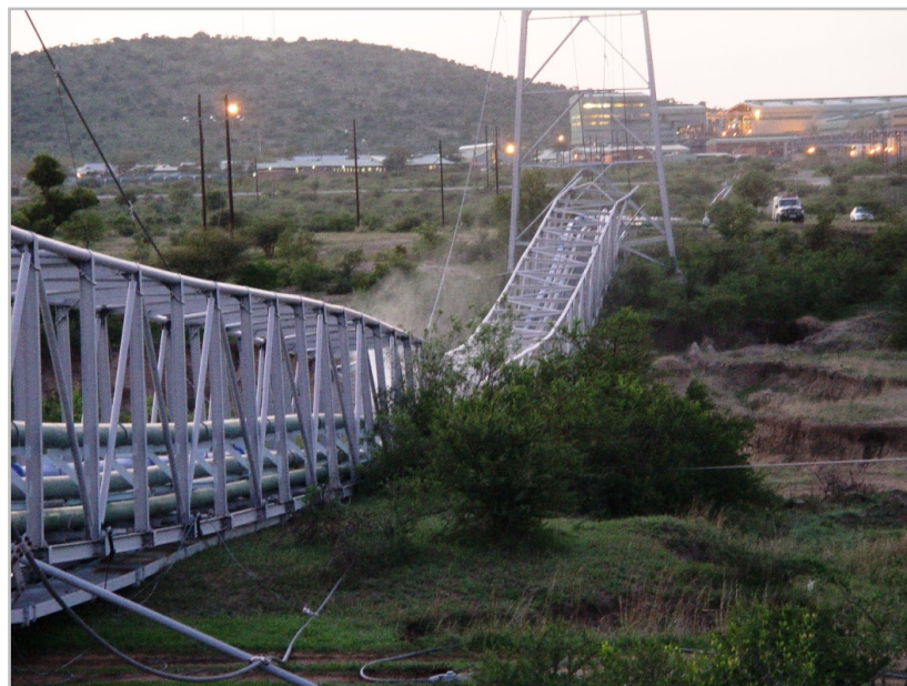
Figure 2.3: Suspension bridge failure due to corroded rope anchors.
