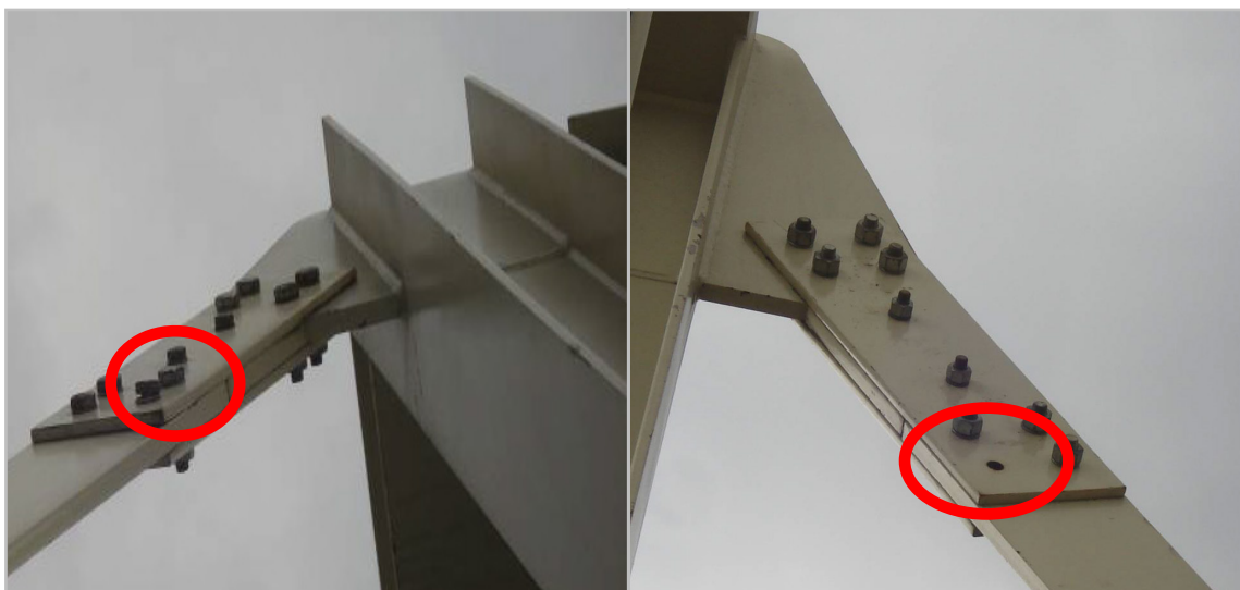
Figure 5.17: Fractured bolt at tie-beam connection months prior to the collapse (14).
