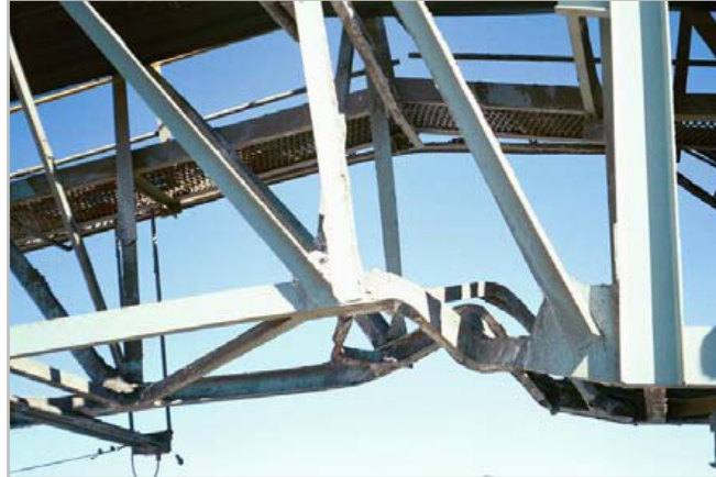
Figure 3.3: Close-up of buckled truss bottom chords.
