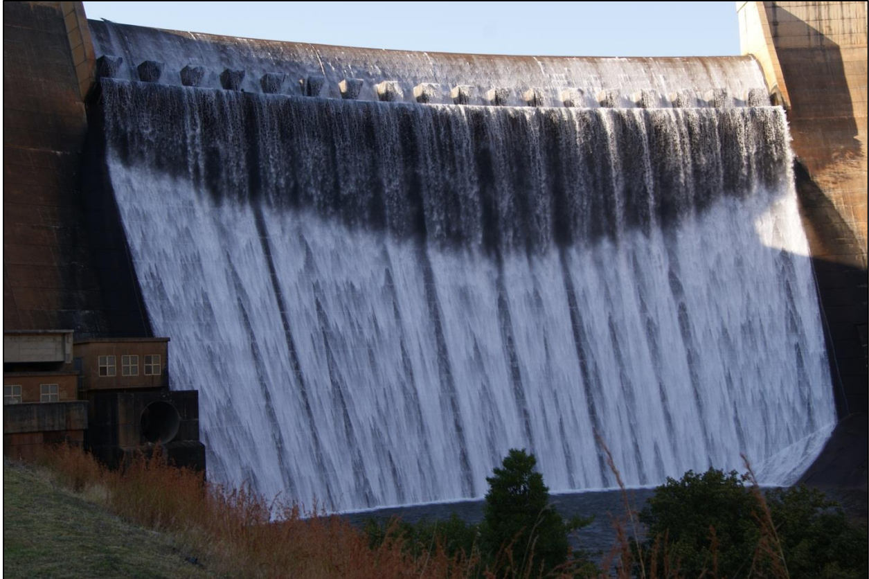
Figure 2-39: Influence of curvature visible at the Blydepoortriver Dam indicating a larger trajectory of water flowing over the center of the spillway compared to the sides.
