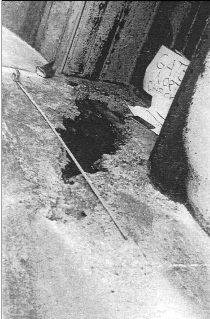
Figure 2-54: Keenleyside Dam cavitation damage on the sluiceway crest near the gate slots (Tatro, et al., 1994)
