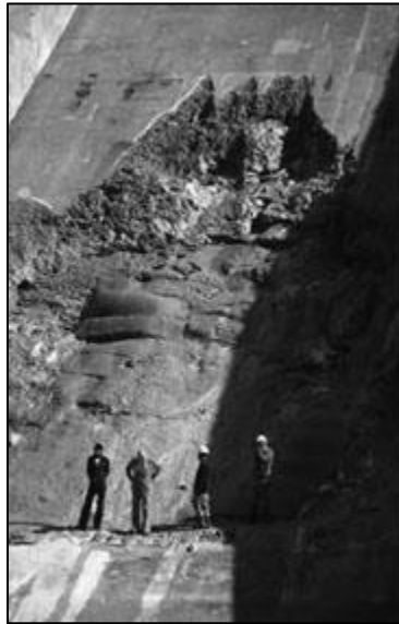
Figure 2-46: Cavitation damage on the Karun dam, Iran (Kramer, 2009)
