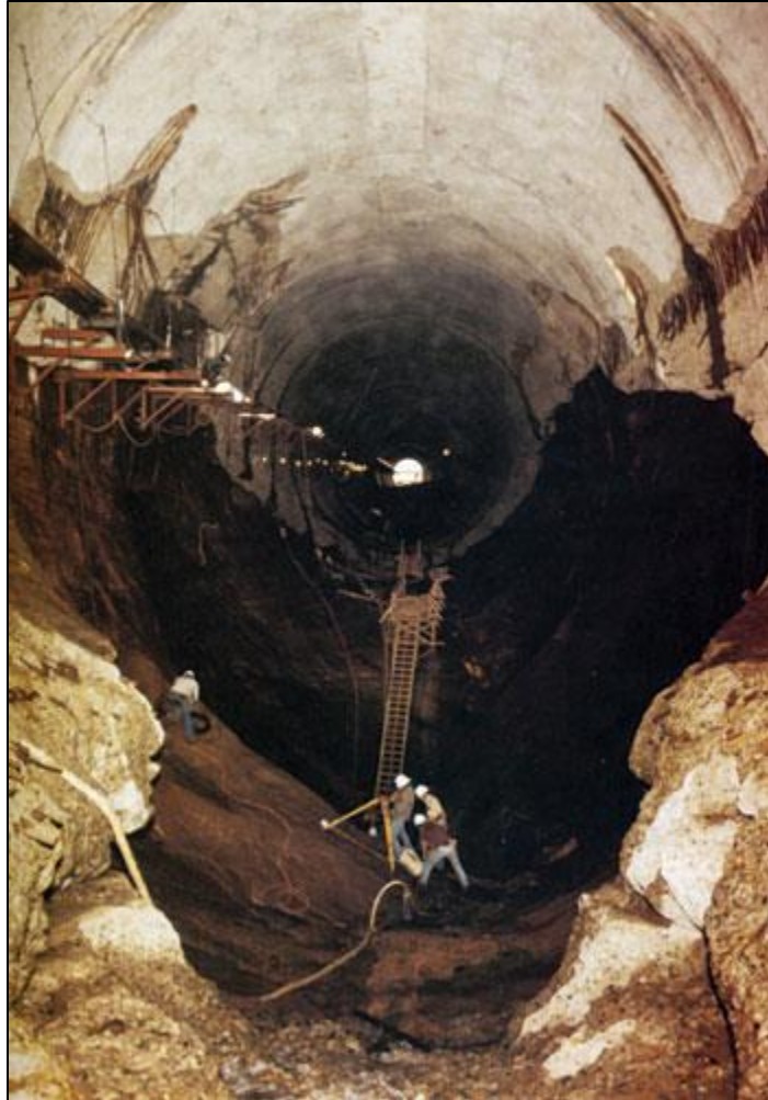
Figure 2-44: Damage in a spillway tunnel at Glen Canyon Dam as a result of cavitation (Morris, 2012)
