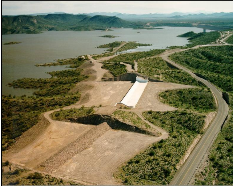
Figure 2-4: Limited service spillway (in foreground) to be constructed and auxiliary spillway (ogee crest) in background at New Waddle Dam, Arizona (LaBoon, et al., 2011)
