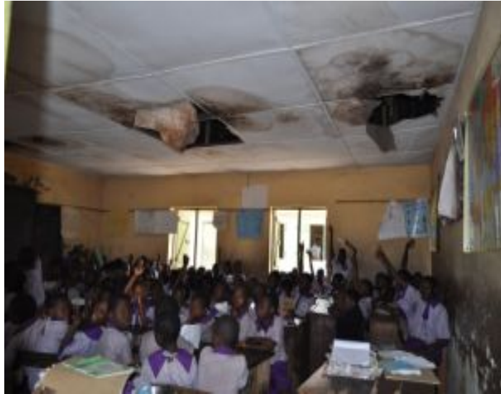
Photo 5.10: The dilapidated structure of the classroom
