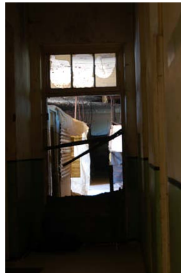
Illustration 44: Rooms in what used to be wards have been divided up into smaller informal dwellings. Sometimes there can be up to nine people living in a small room (Author, 2012).
