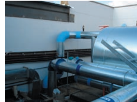
FIG. 5.3.4.5.1 Chiller plant on roof of new Law Faculty, University of Pretoria
