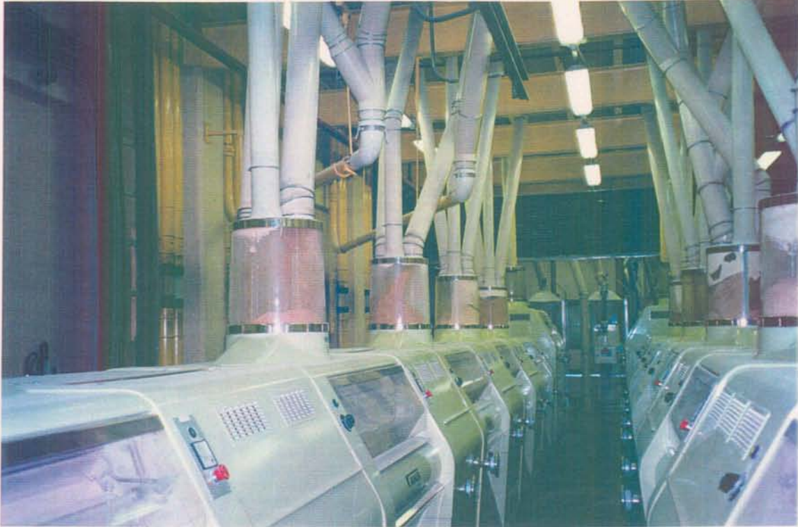
Fig. 3: Part of a roller floor in a South African mill
