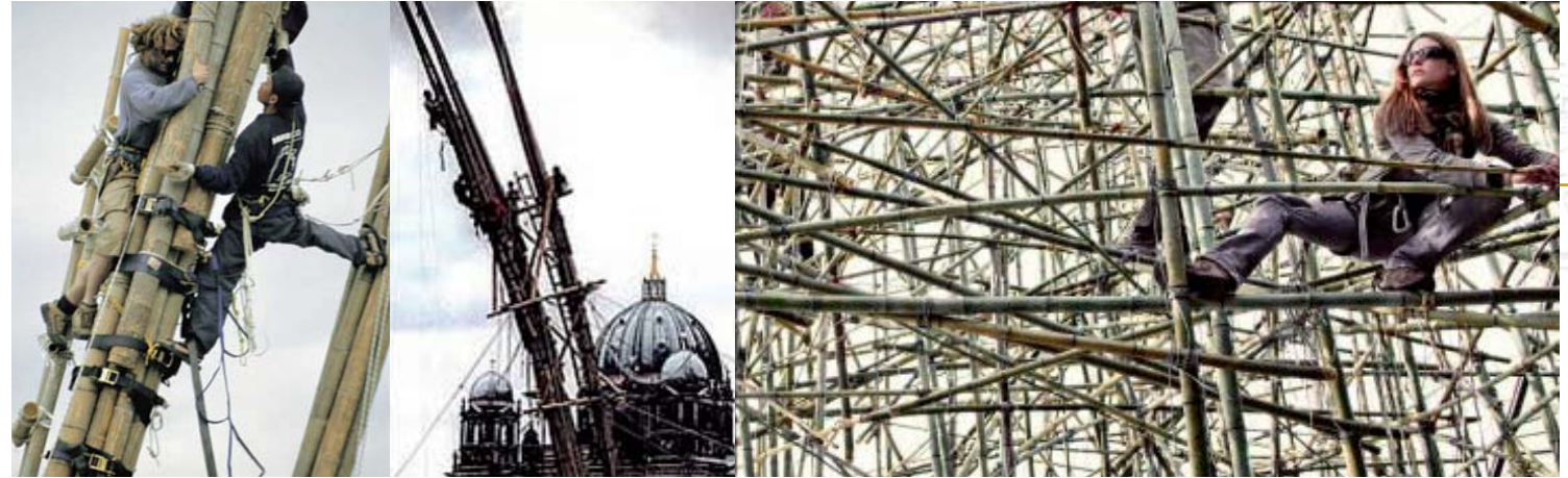
Figure 122, 123, 124: Live building workshop as testing ground for bamboo construction for South Africa.
