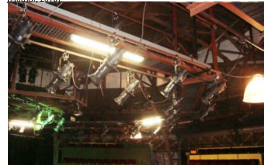
Figure 143. Lighting system in the Main Theatre fixed to the existing roof structure (Author, 2010).
