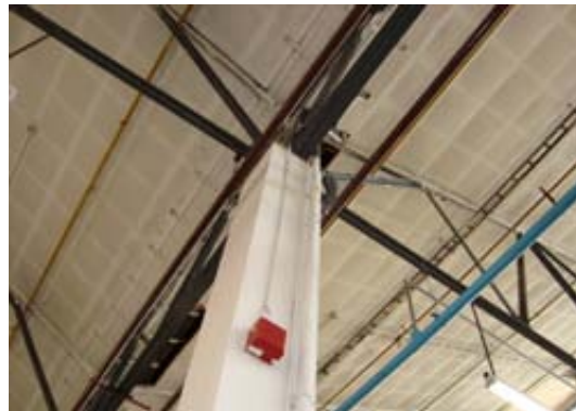
Figure 79. Steel truss supported by column. Note the water pipe, electrical cables and sprinkler system supported by the truss structure (Author,2010).
