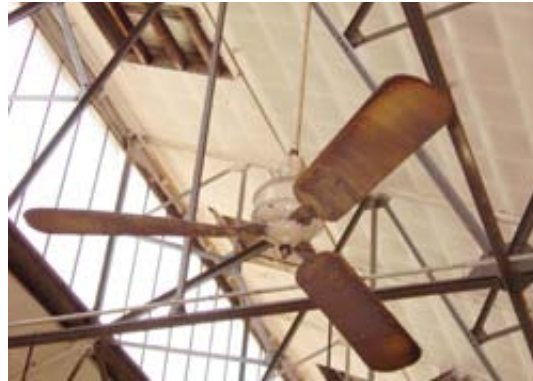
Figure 84. Existing electrical fans (Author,2010).
