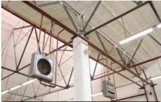
Figure 86. Existing ventilation system (Author, 2010).
