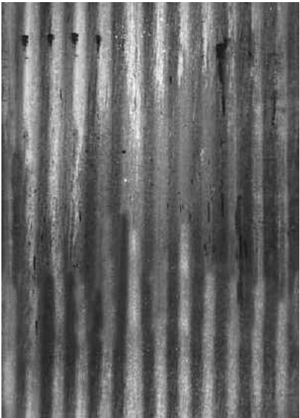
Fig 6.26 Profiled sheeting is used as a roofing material. It is also used as cladding for the traders stall
