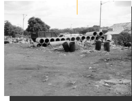
Fig 1.20 Dump on the site
