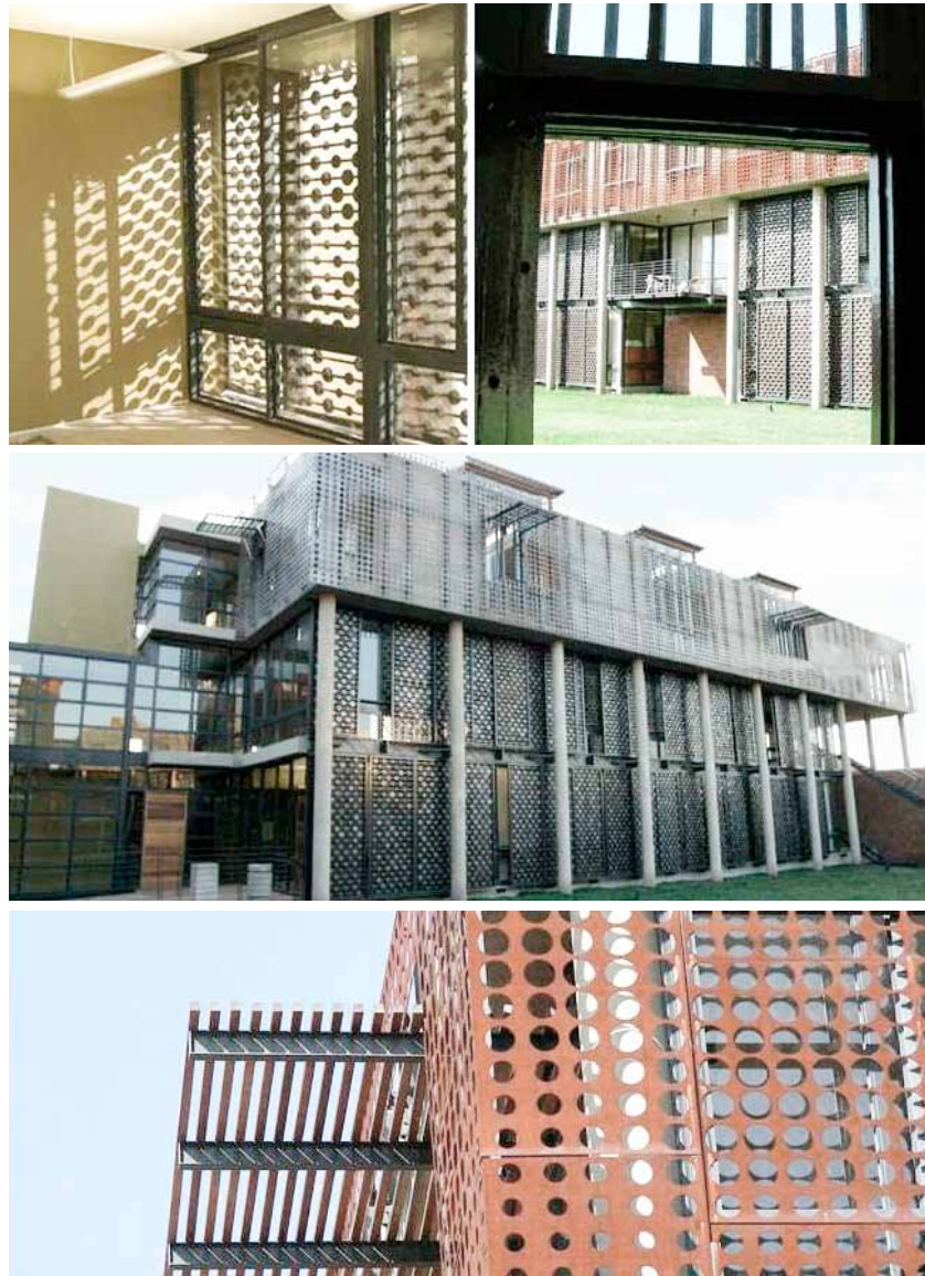
Figure 5.5: Collection of images of the solar screens at the Woman's Jail Precinct, Constitution Hill. (Kate Otten Architects, 2007)
