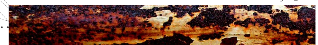
fig 89 g_. Rust and paint.
