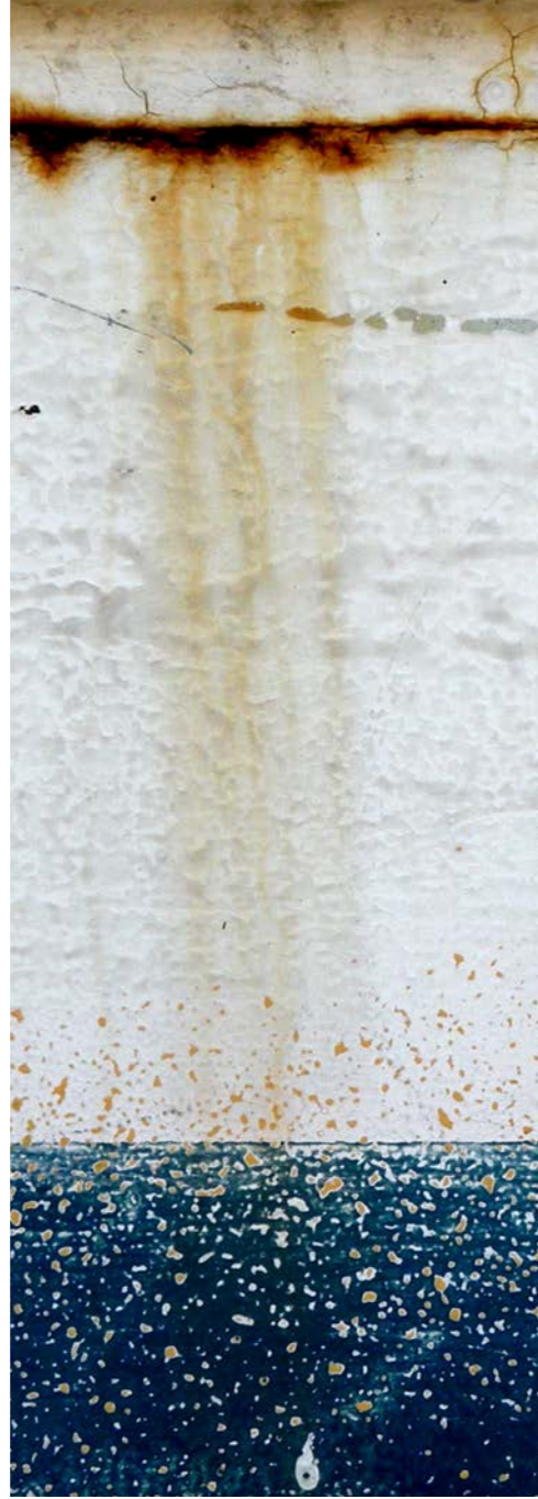
fig 97 c. Rust stain.
