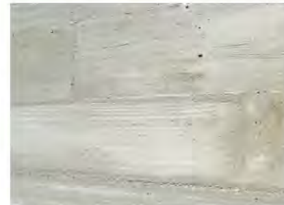
fig 159. Rough sawn off shuttered concrete (google images)
