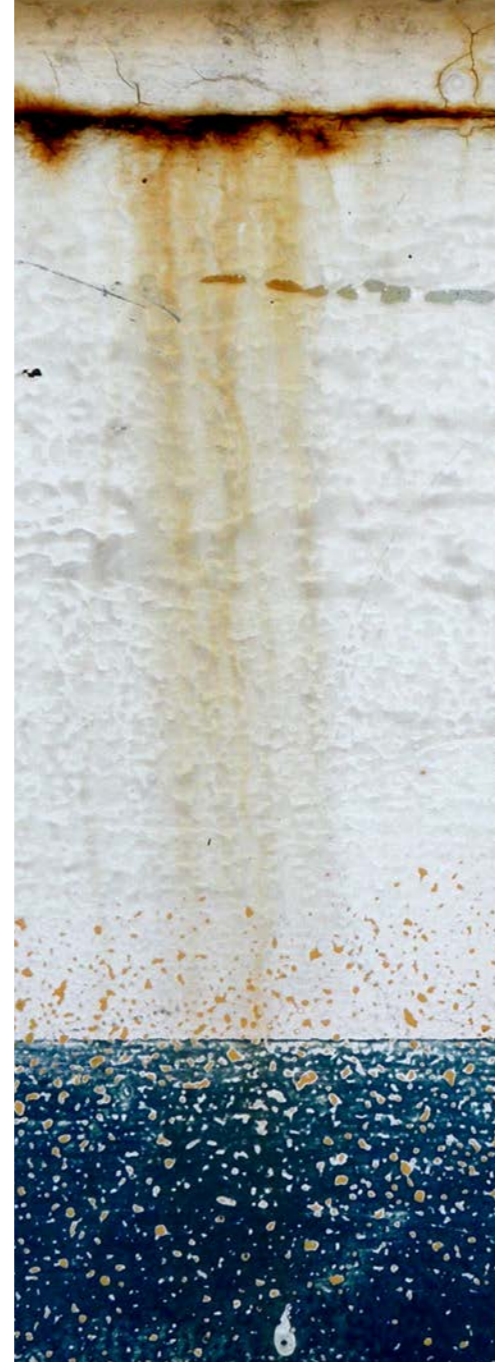
fig 97 c. Rust stain.
