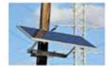
ELECTRICAL SUPPLY IN SOLAR PV CELL
