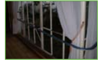
Handrails to prevent injuries at windows
