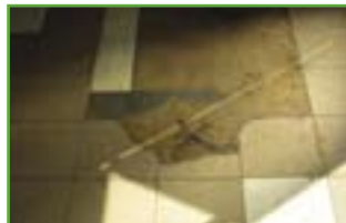
Change in floor level can cause accidents
