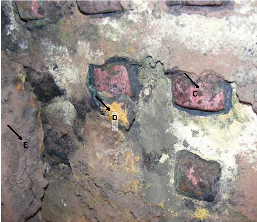
Figure 4: Detailed view of the copper waffle knobs; C = copper waffle knob; D = corrosion product with ramming material; E = freeze lining (FL).
