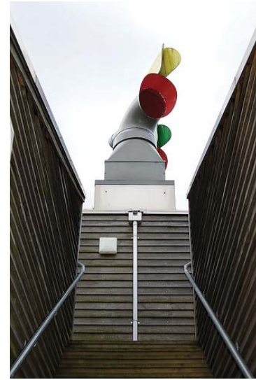
Fig.232:Wind driven ventilation system in Sutton, England. Wind cowls use the wind to draw warm stale air up from inside, and direct fresh air downwards over passive heat exchanger [Source: www.flickr.com/photos/8586443@N03/2377282168/in/photostream/ ]
