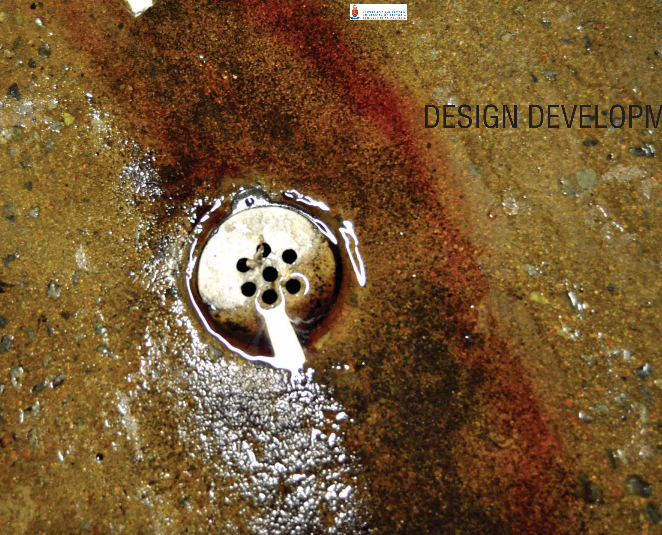
Figure - 8.1 - Photograph of a floor drain in the Rietvlei Abattoir (By Author).
