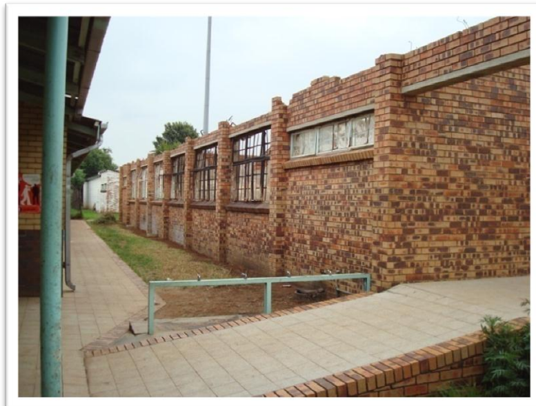
Figure 4.5: Burnt classroom block at Mr Sogo' school
