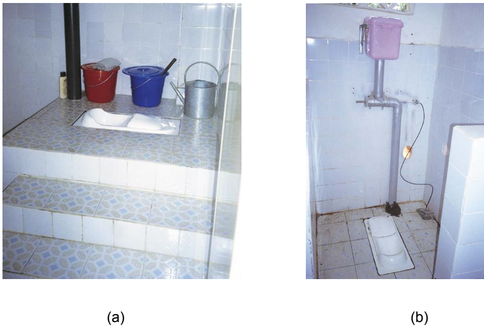
Figure 2.14. Urine-diversion ecosan toilets in Nanning area, China.
