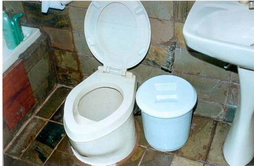
Figure 2.27: Retrofitted urine-diversion toilet in Richard Holden's house in Bellevue, Johannesburg (Photograph: CSIR)
