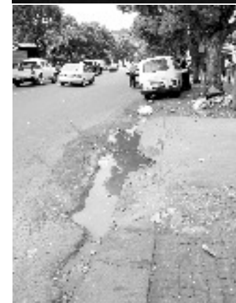
Fig.4.8 Struben Street - dirty and wet, a pedestrian-unfriendly strip
