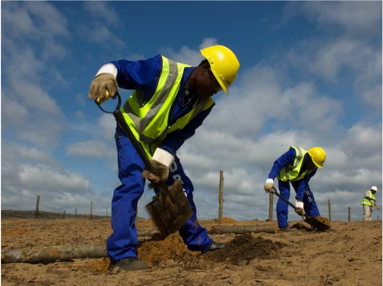
Plate 1-2. This plate shows a rehabilitating site at less than 1 year old. Topsoil stockpiled prior to mining is replaced on re-shaped dunes and wind-breaking fences are erected to limit soil erosion. The soil is seeded with exotic annual seeds that provide a cover crop, further stabilising the soil. The photograph was taken by Prof. R.J. van Aarde and is used with permission.
