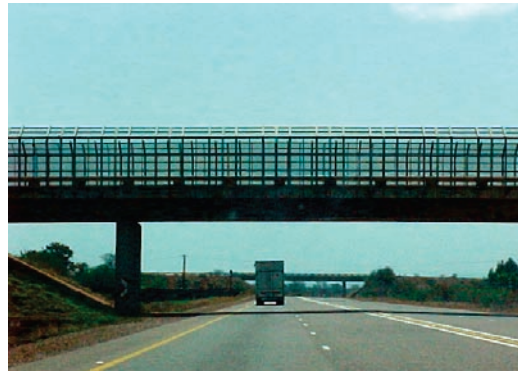
Figure 4.8 A bridge connecting two informal settlements crosses the N1 - a common element sighted throughout the journey from Pretoria to Makhado. The concrete and steel bridge is clad in profiled channels and steel mesh to stop people throwing objects at passing traffic
