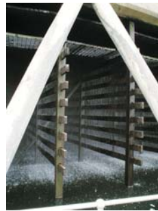
fig 5.5 Ground floor of cooling towers
