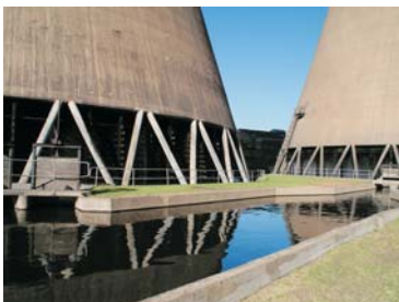
fig 5.7 Water channel leading to cooling towers
