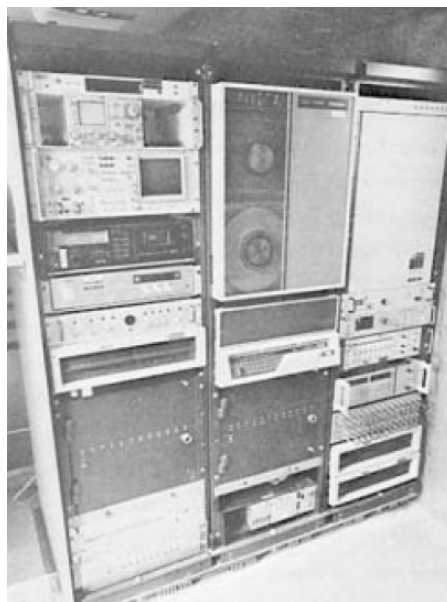
Figure 2.2: Equipment rack of an MIT mobile vehicle DSN node [13].
