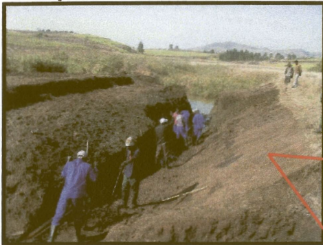
Figure 140: Headcut erosion feature. Geocell chute preparations.
