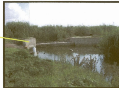
Figure 3: Concrete weir at site 4. Note the wetland vegetation (tall emergent, Phragmites australis ) behind the structure.
