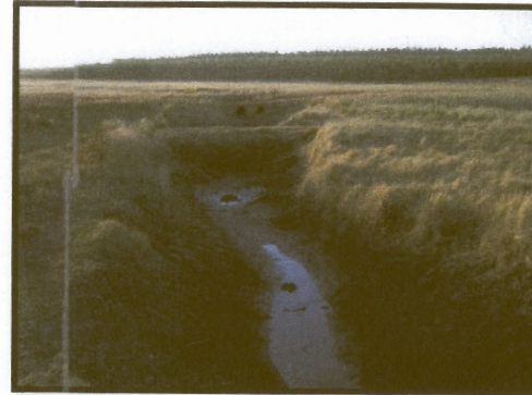
Figure 26: Drains with clay plugs and evidence of wetness. Photo taken 26/05/2003.
