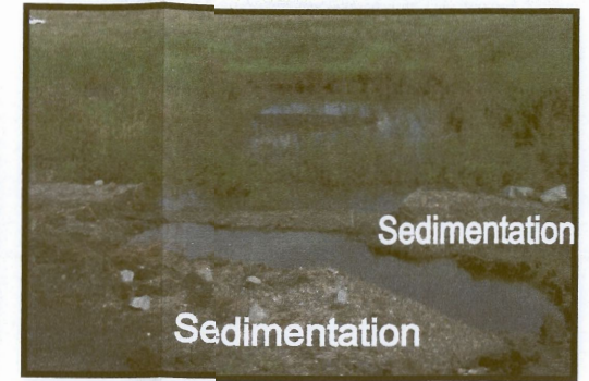
Figure 131: Site no 5.1.. Sedimentation taking place behind the structure.
